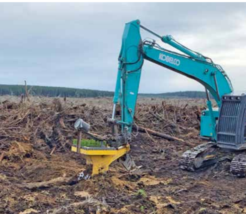
Figure 4: Mechanised planting in Kaingaroa Forest using the M-Planter. Photo courtesy of Ben Dixon, Timberlands
