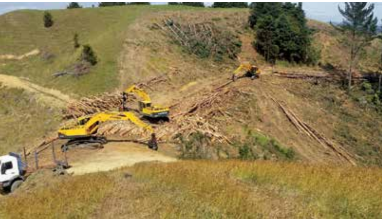
Bent Fish Gully with the processing machine in the centre. An off-road truck loading machine is temporarily shovelling in the background. The felling machine has been shovelling from the right (out of picture) and is about to load an off-road truck which is reversing into position
