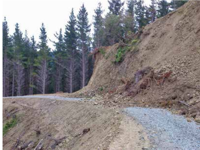
A cut slope on a newly-constructed road that has slumped following a rainfall event in Gisborne
