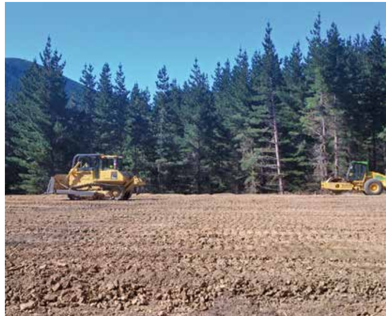
Summertime landing construction in Canterbury. Compaction involved track rolling the landing with a Komatsu D65 EX bulldozer (left) prior to vibratory rolling with a Sakai SV512TF (right)
