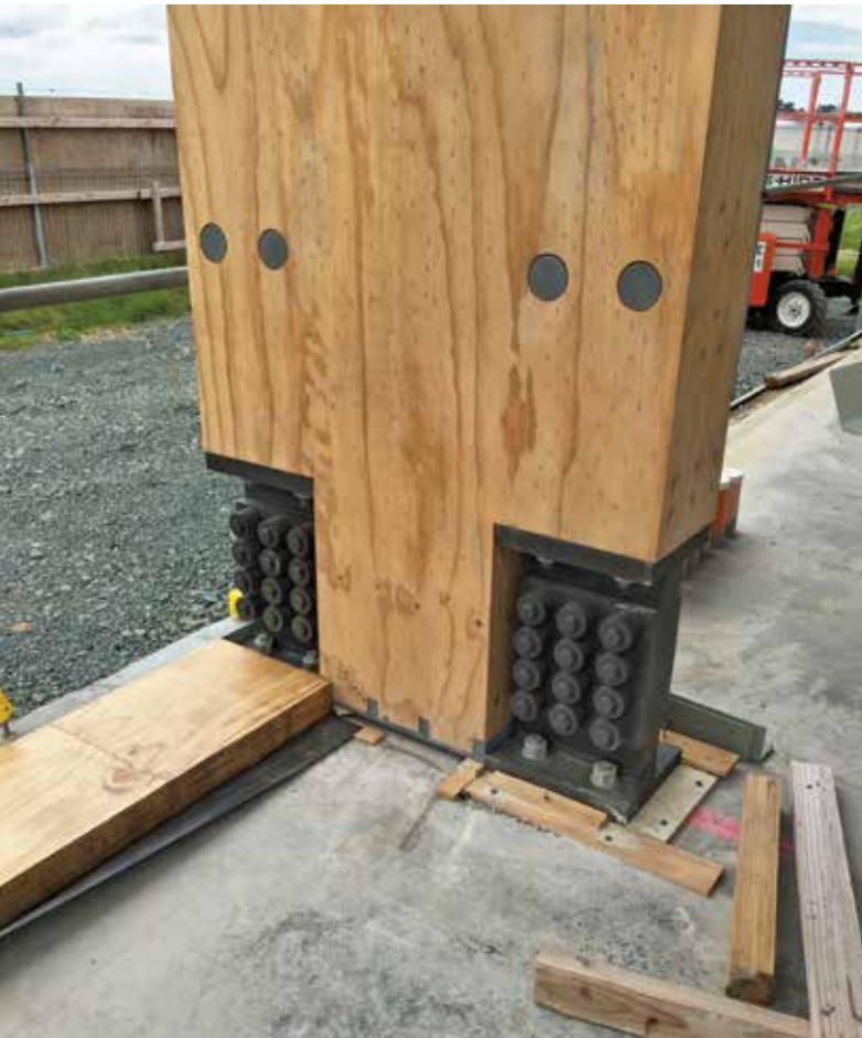
1200 x 300 mm LVL column with two RSFJs connected at the base building project conducted for Airways NZ rather than Nelson Airport.
