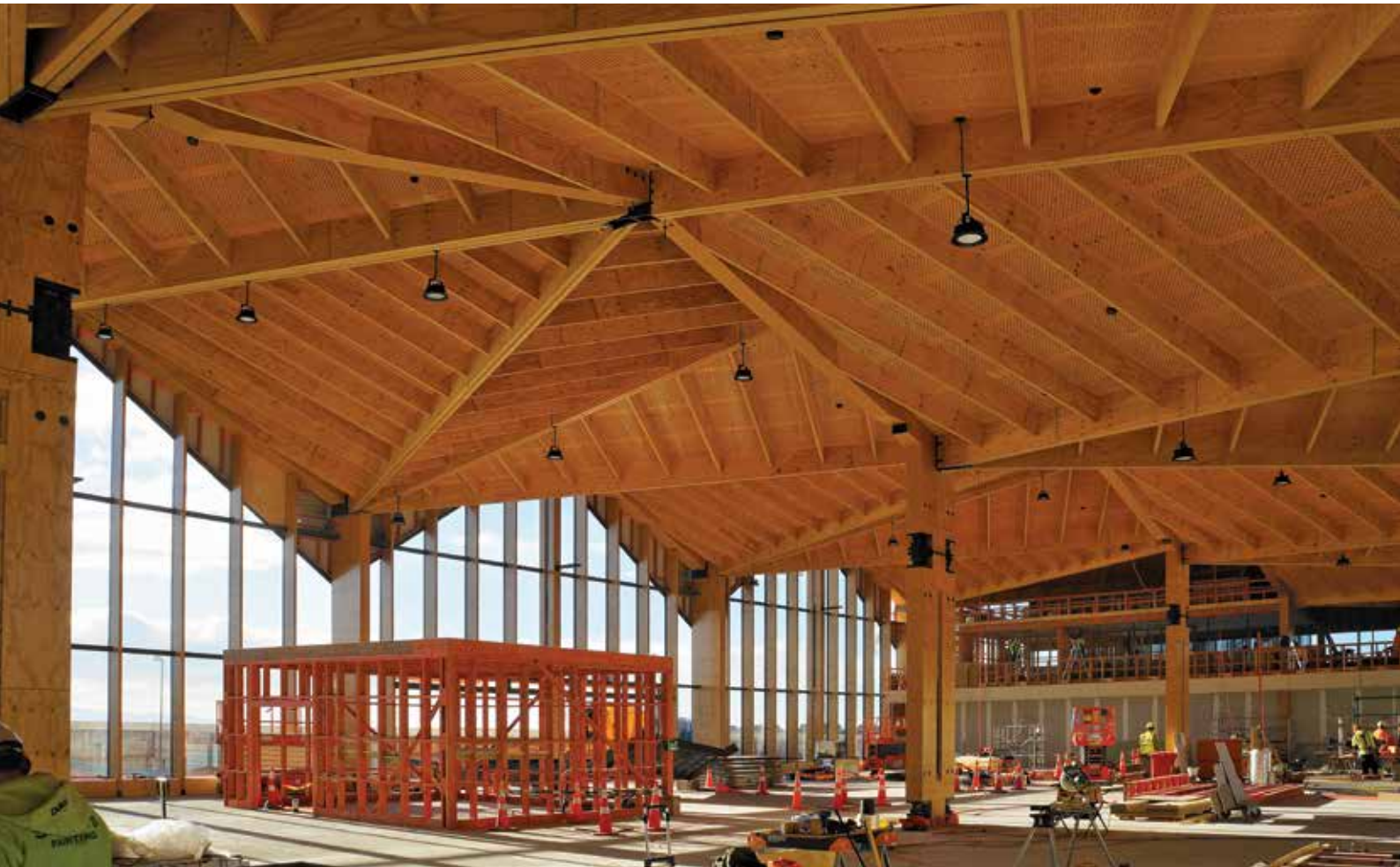
Engineered timber in the Nelson Airport Terminal under construction. Photo courtesy of David Evison
