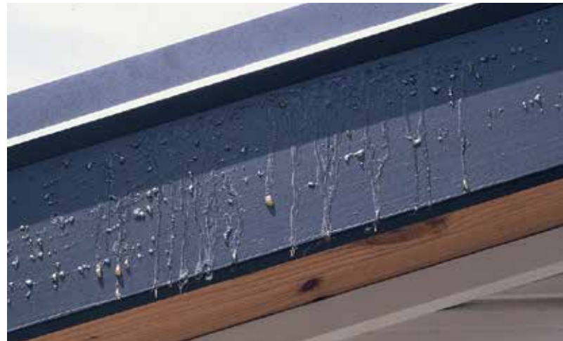
Resin show through in a painted fascia board. Source: Scion Digital Image Library
